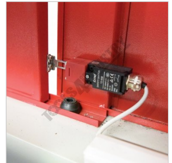
Rear Doors Safety Micro Switch
