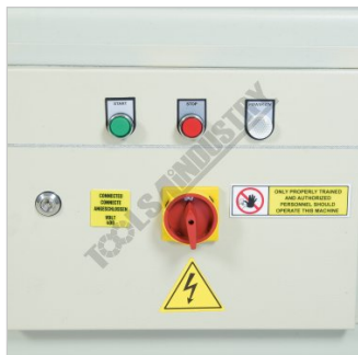
Main Power Control Panel & Isolation Switch
